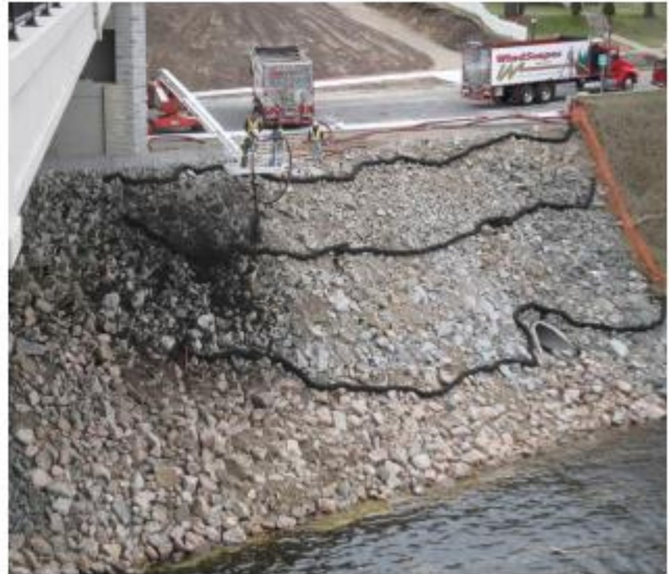
The TH 23 Mississippi River Crossing project was installed during in the fall of 2009.
